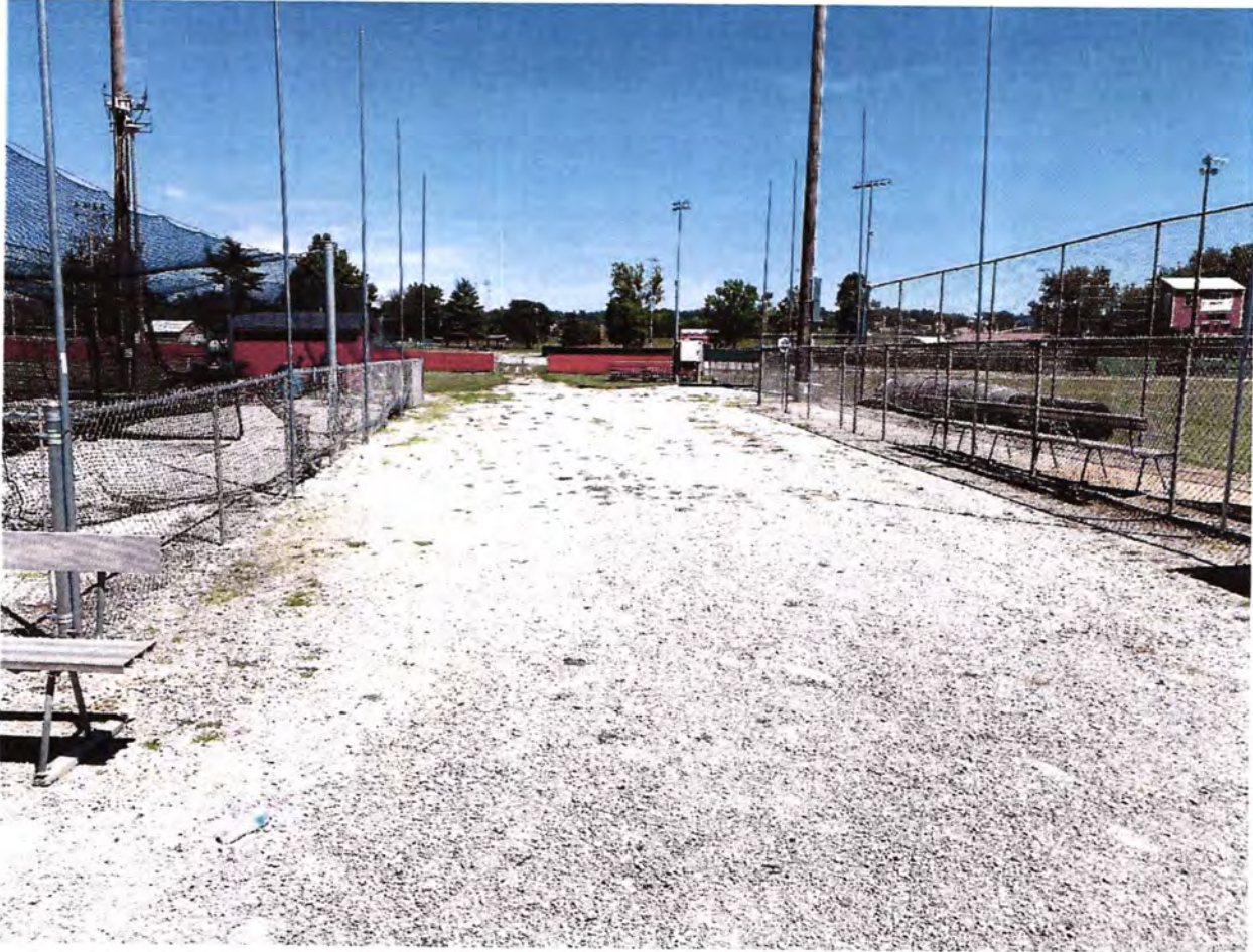
Additional gravel needed to fill worn out areas and weed control.
