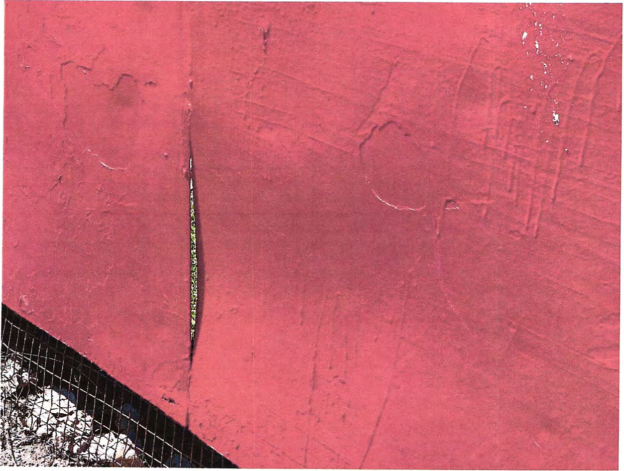
Outfield fence coming apart.
