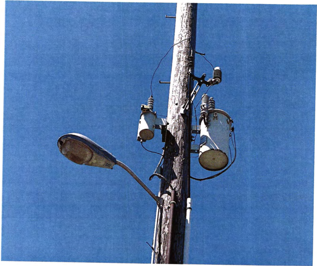
Overhead exposed wiring on light pole from transformer. When it rains, the wiring sends sparks to the ground.
