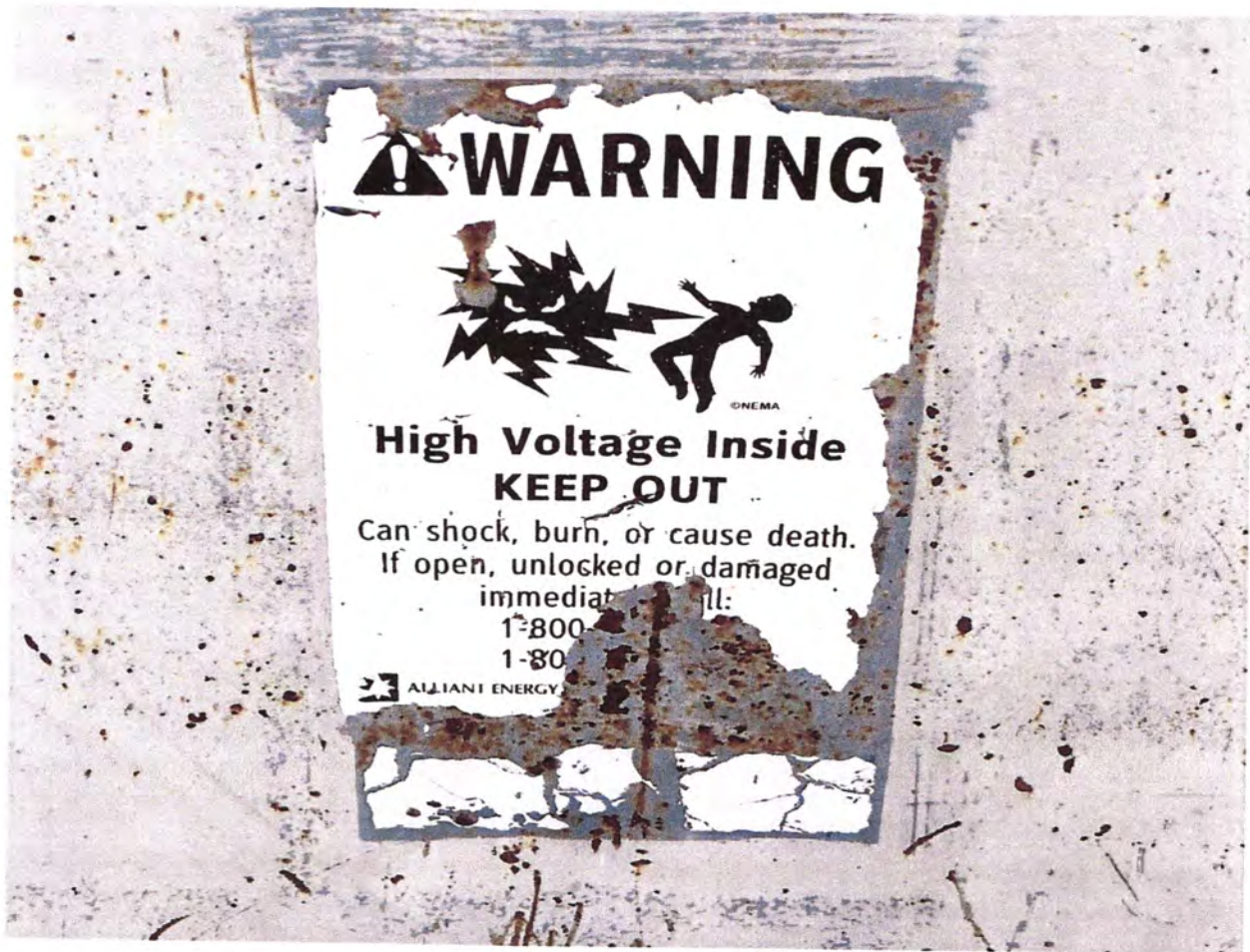
Picture of High Voltage warning sign on Transformer box.
