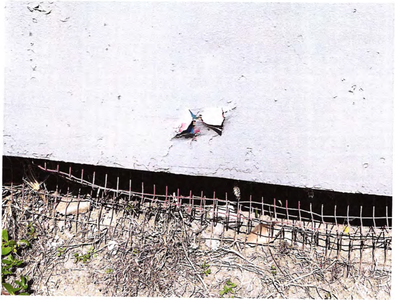
Hole in fencing
