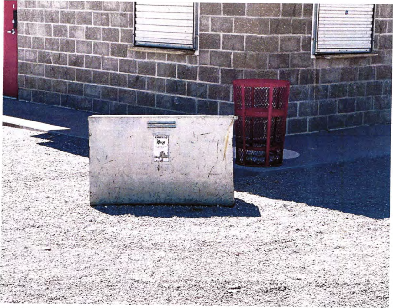
High Voltage Electrical Transformer in front of concessions.
