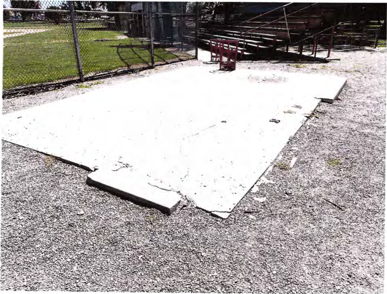
Cracked and broken concrete we need to repair
